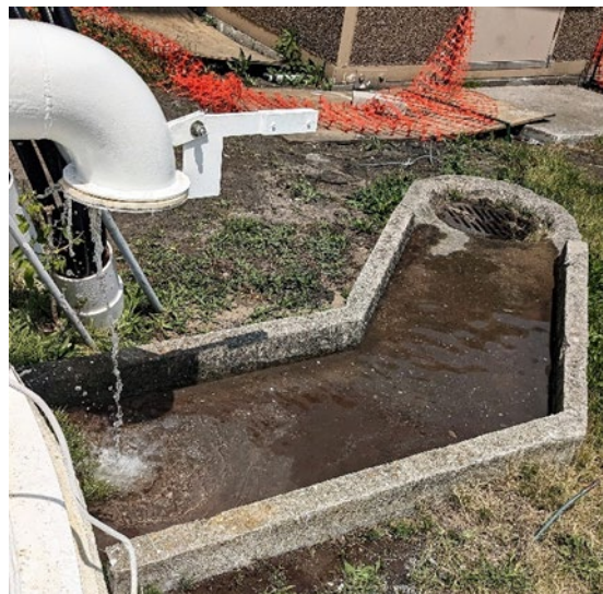
Water Overflow at the M-32 Water Tower
